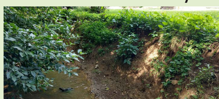
Hubers Run was relocated in the early 20th century and currently drains to the Litz Run at the Woodstream complex within Litz Borough. The relocation along with encroachments by landowners into the floodplain has contributed to the steep banks and increased erosion.
